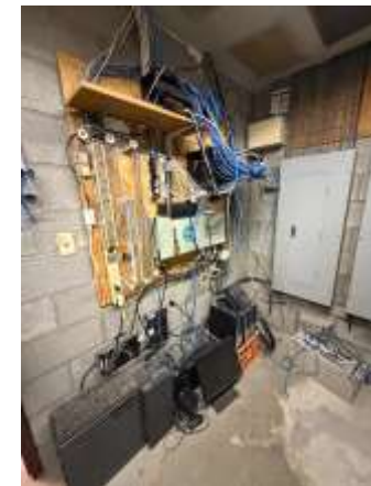
Existing communications/network equipment and cabling area.
